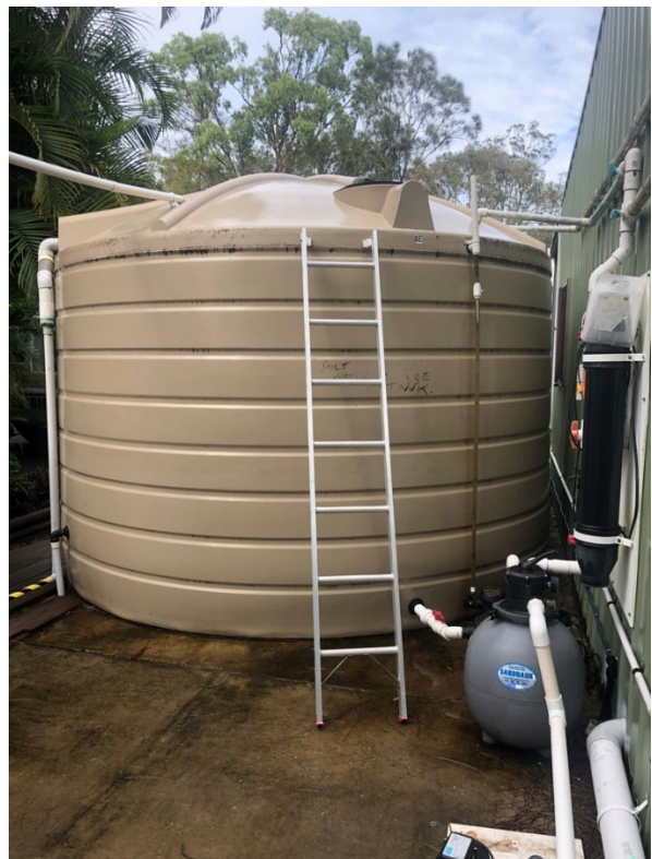
The 20,000-litre storage tank
